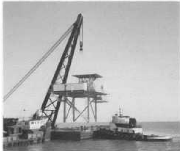
PRODUCTION DECK for SMI 253 platform being offloaded from cargo barge for installation on submerged gravity base.
