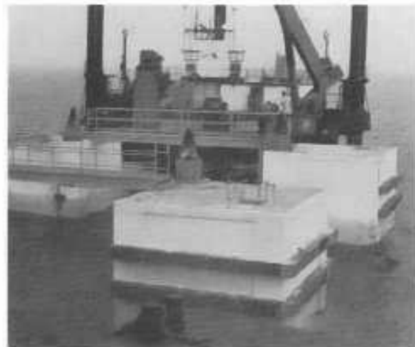
GUIDE CONES on gravity base guide deck legs into place before final welding.
